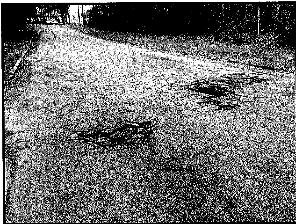
Photograph 5 – Deteriorating Pavement on Fairington Drive Adjacent to Site
